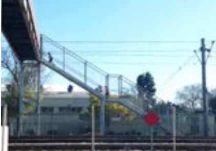
The only pedestrian bridge crossing over the Blue Line and railroad tracks at Roosevelt Park is used for fitness training and could be renovated to be a positive visual landmark in the community.
